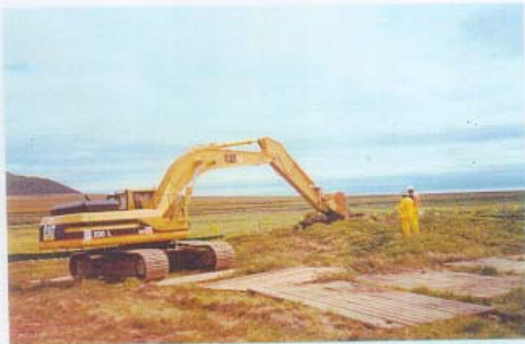
Figure 3-3: Excavator Removing the Surface Vegetation Getting Ready to Start the First Lift – 1993.
